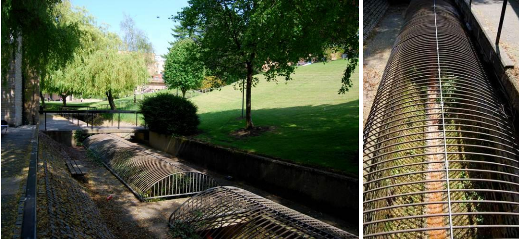
Figures 10 & 11: The caged over stretch of Westbrook in the north western pocket of Bradford University. Source: Michael Canning 2012
