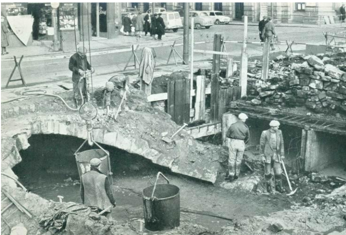
Figure 9: Bowling Beck, construction of new culvert March 1964, the exposed masonry is Cuckoo Bridge built in late 1700's. Source: Telegraph and Argus.
